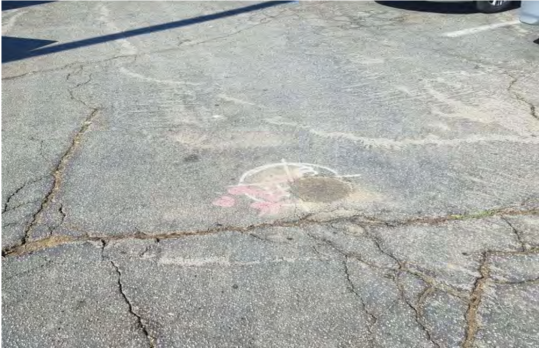
Geo -Technical Boring Patched
